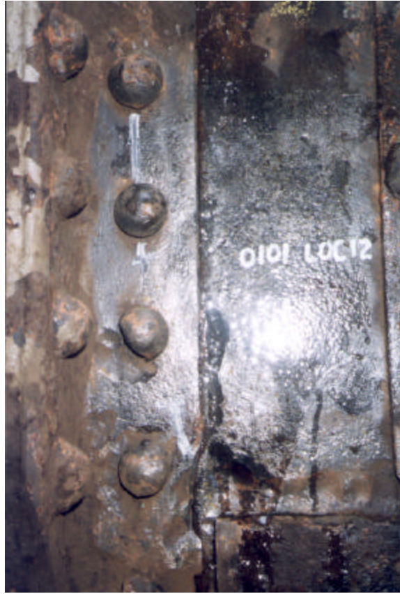
Figure 2. Ultrasonic scanning results of the same location as shown in Figure 1. Note the location of the crack beneath the connection angle, ending between the fourth and fifth rivets.
