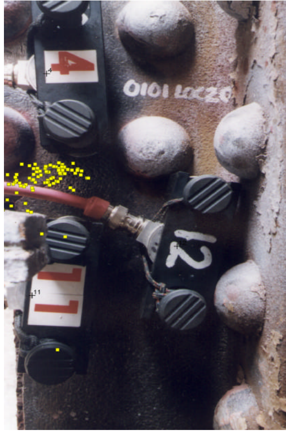
Figure 4. AE monitoring results from a crack originating in the cope of a floor beam connection angle. PT inspection confirmed that the tip of the crack was at the center of the cluster of located AE events.
