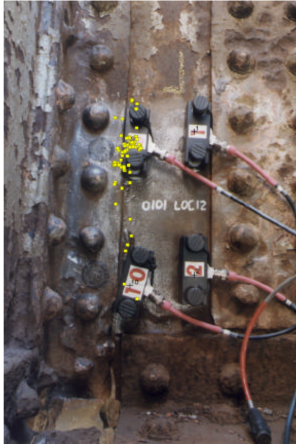
Figure 1. A cluster of source located AE events, with crack growth characteristics, between the fourth and fifth connection angle rivets.
