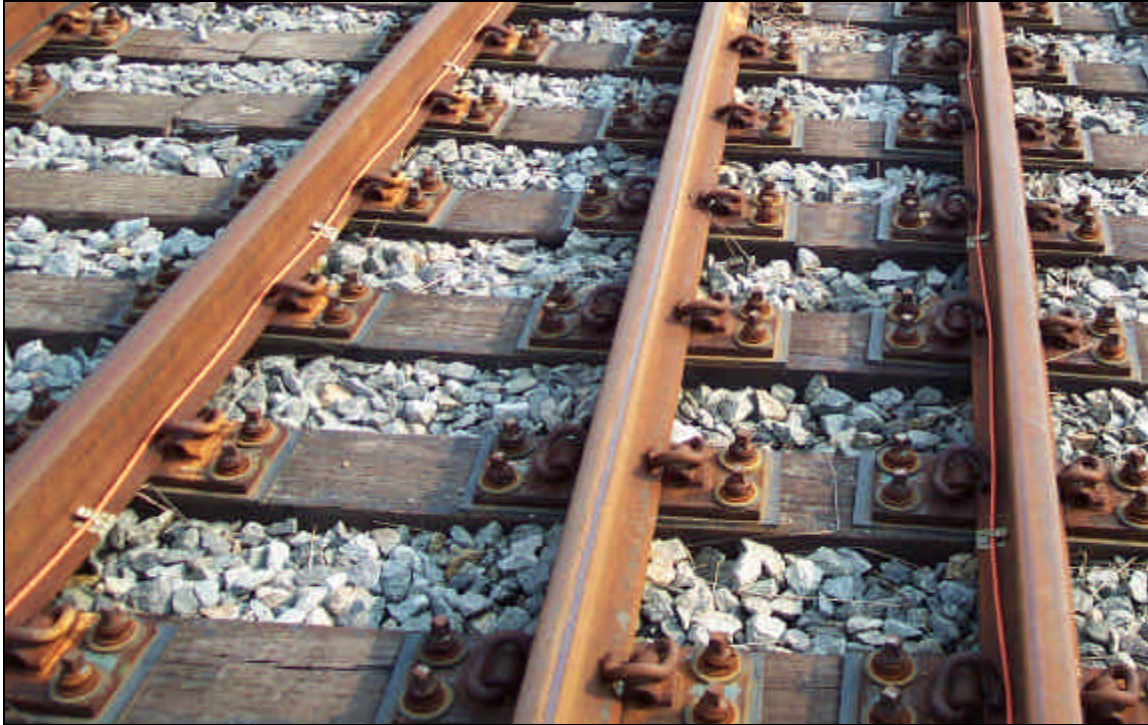
Figure 13 – Fastening system on wood ties used for isolating stray current
