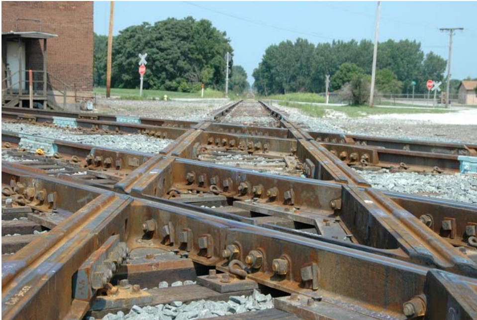
Figure 3. OWLS Diamond in place, Walkerton, Indiana
