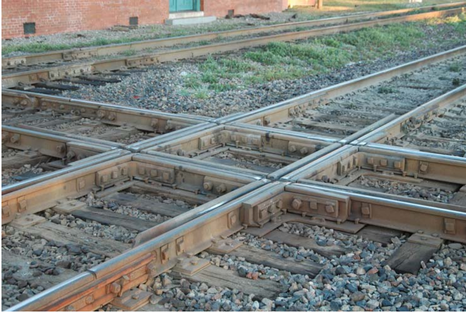
Figure 1. Conventional 3 rail diamond in place nearing end of life cycle. Plant City, Florida.
