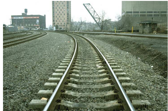
Figure 3-5 Concrete Ties – Photo by Kevin Keefe
