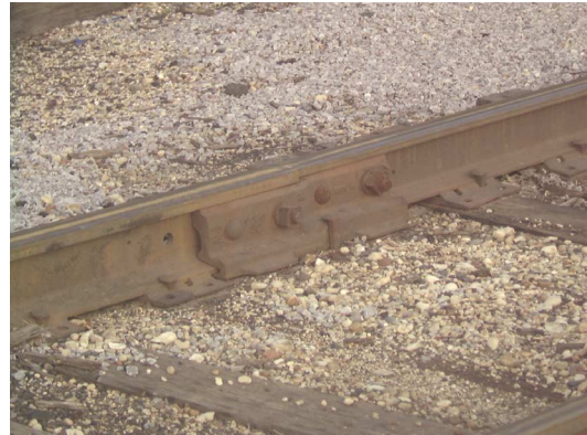
Figure 3-10 Compromise Joint Bar – Photo by J. E. Riley
