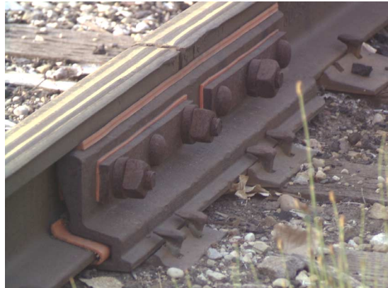
Figure 3-11 Continuous Insulated Joint – Photo by J. E. Riley
